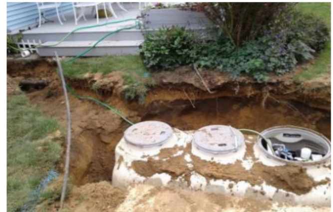
Innovative/Alternative Onsite Wastewater Treatment System Installation (Fuji Clean CEN Series) - Photo Credit: Suffolk County
