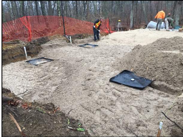
59 River Road (Unlined System)
