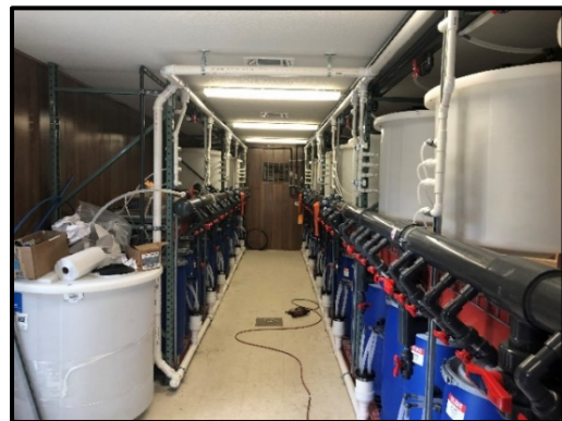
Overall View Inside Column Trailer
